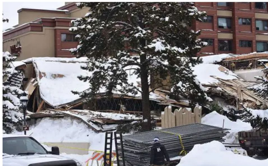
The roof of the Ten Mile Room in Breckenridge collapsed from heavy snowfall Jan. 11, 2017.
